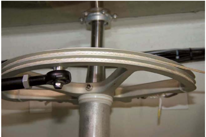
Steering quadrant – all cables should be adjusted and checked for any excessive wear.
