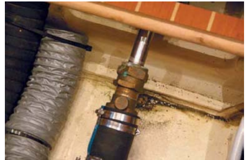
Stuffing box – Stuffing boxes should be checked for excessive leakage. A slight drip is normal. Excessive dripping indicates either adjustment or repacking of the unit. A "normal" drip rate is often considered about 4-5 drops per minute. This should be checked as part of a sea trial.
