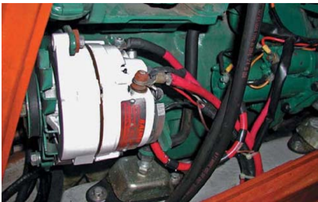
Alternator and starter motor terminals – should be protected with insulating boots. NOT as shown here. Remember that the starter motor circuit is the only circuit on a boat that is not required to have a fuse installed. If a metal object contacts the terminal and the engine block simultaneously, a serious short circuit will occur, possibly causing an engine room fire.
